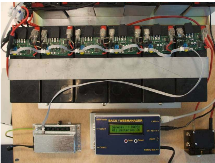
Figure 13: BACS System installation
